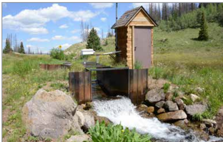
A Parshall flume measuring the flow of the Tabor Ditch at Spring Creek Pass, one of the 40 or so active diversions of water from the west side of the Continental Divide to the east side. CLUI photo
