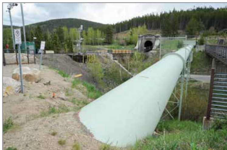
Pipeline emerging from the ground then entering the Moffat Water Tunnel, next to the west portal of the Moffat Train Tunnel. CLUI photo
