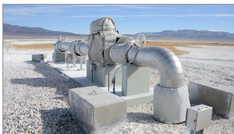
Recumbent waterpipes at Owens Lake.
